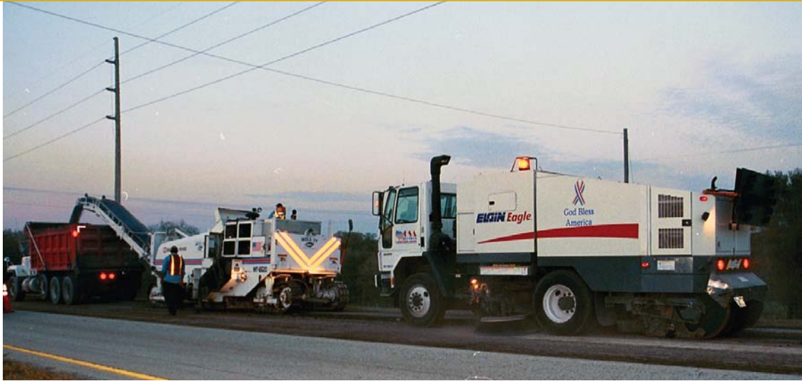
An Elgin Eagle sweeper cleans up after a road-milling machine during a road resurfacing project.
